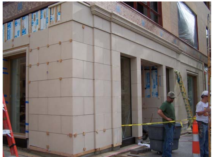
Moldings and Veneer Panels Burberry, Kansas City (Photo shows installation in progress)
